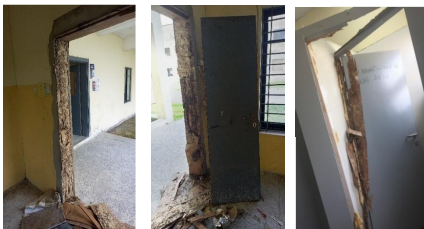
Plate 2A, B and C. IndoorTermite Damges to doors & door frames at CHS from Macrotermes attacks.
